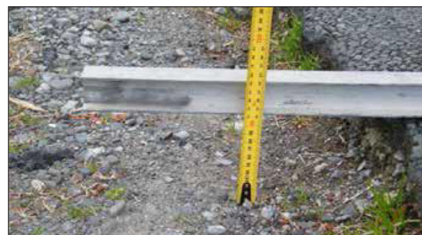
Drop greater than 100mm not acceptable.
