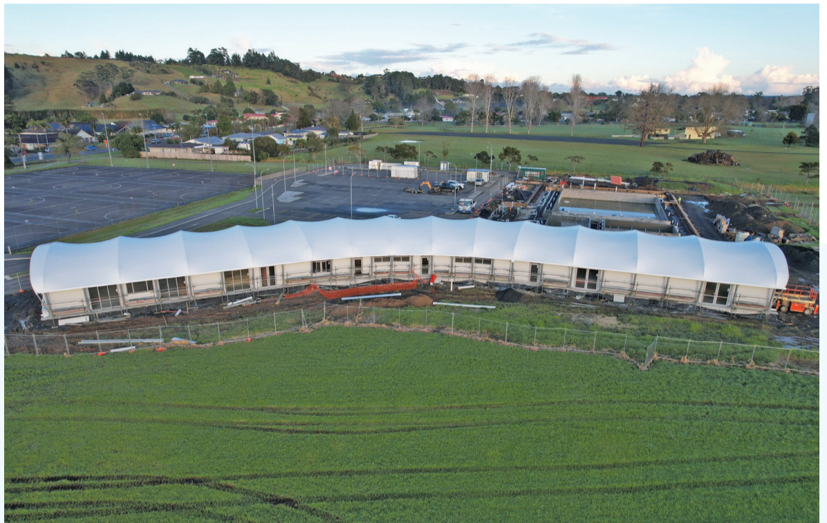
You can track construction progress at Te Hiku Sports Hub Aquatic and Sports Facility on the project Facebook page.
