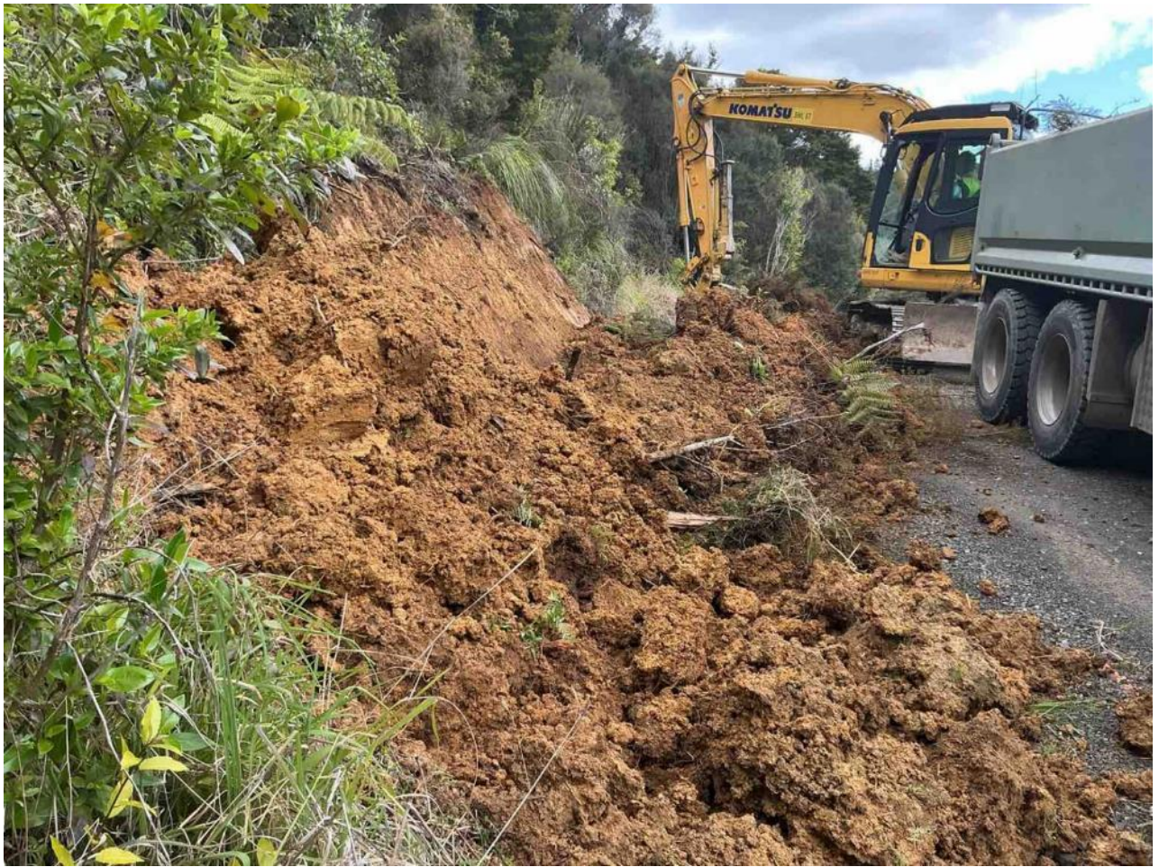
Humpfreys Rd – Slip retreat in progress
