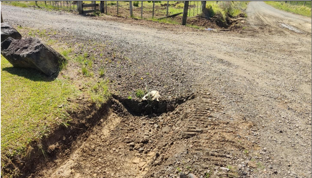
4. Non functioning culvert under vehicle crossing
