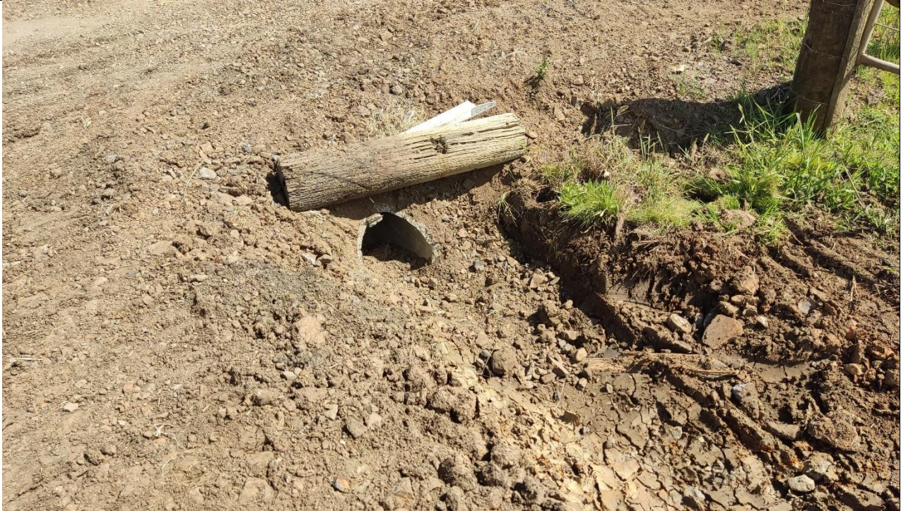
3. Non functioning culvert under vehicle crossing
