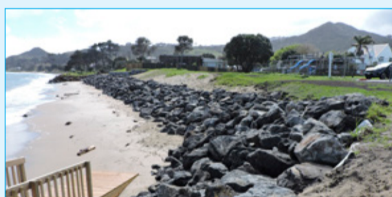
The new seawall and beach ramp are now in place at Freese Park.
