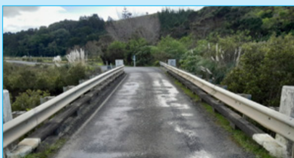
Restrictions at Hihi Road bridge will be in place for six weeks.
