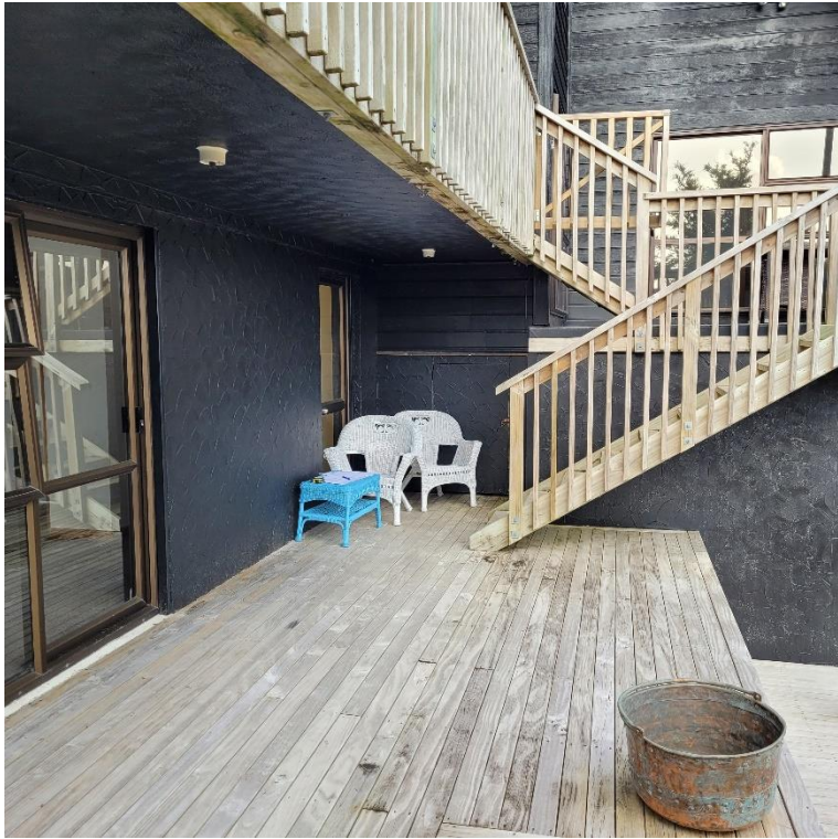
Common deck on lower level (L3), water pump is accessed from here.
