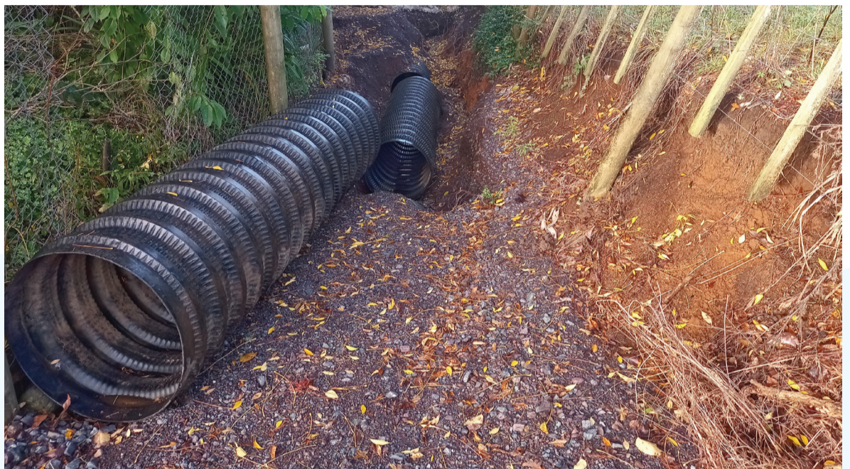
Works include increasing the stormwater capacity of the track to Charlie's Rock.
