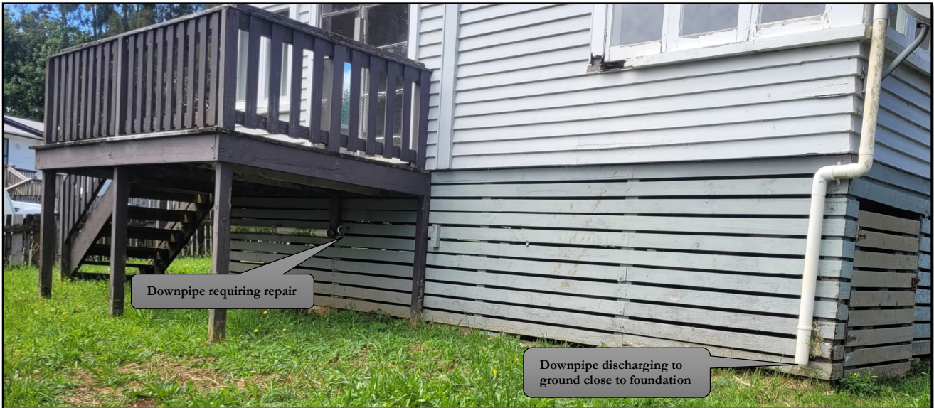
Figure 8: Downpipes requiring repair and/or connection to existing stormwater infrastructure for the proposed Lot 1
