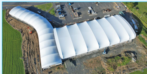
The roof over the aquatic wing at the new facility is completed.
