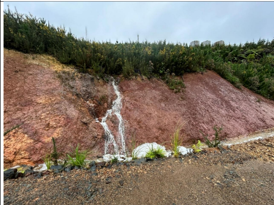
Photo 20: East-facing view of the bottom of the discharge field where significant buildup of white foam is visible. Condensate runoff from the field flows along a channel in a southern direction.
