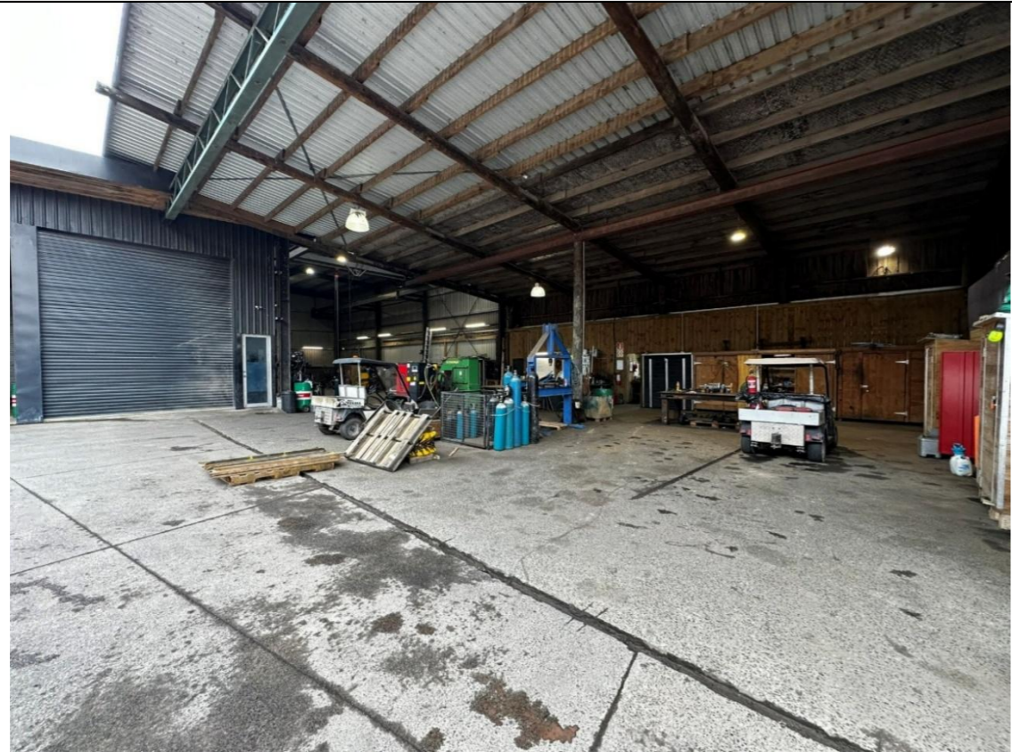
Photo 1: Minor staining visible in the middle section of the engineering workshop.
