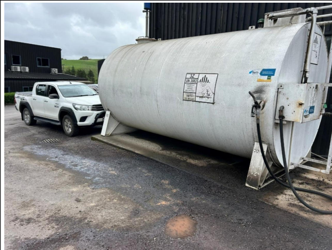
Photo 12: View of the diesel AST. Spilled diesel is visible flowing towards the stormwater drain.
