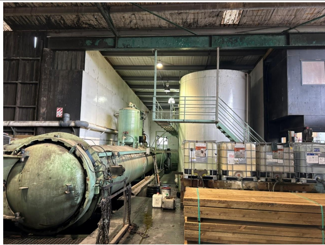
Photo 3: The treatment area within the main timber treatment plant consisting of the treatment cylinder, chemicals stored in IBCs and the mixing tank.
