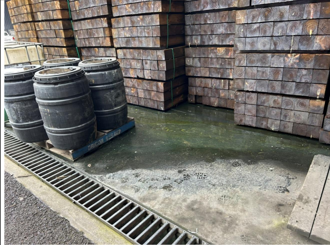
Photo 5: Green chemicals and staining observed on the drip pad.
