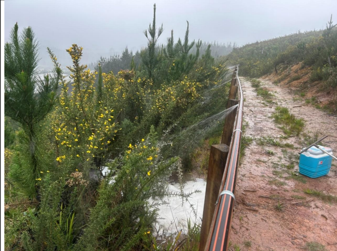
Photo 18: Active spraying of condensate onto the discharge field from the drip lines. Foam buildup was observed under discharge points.
