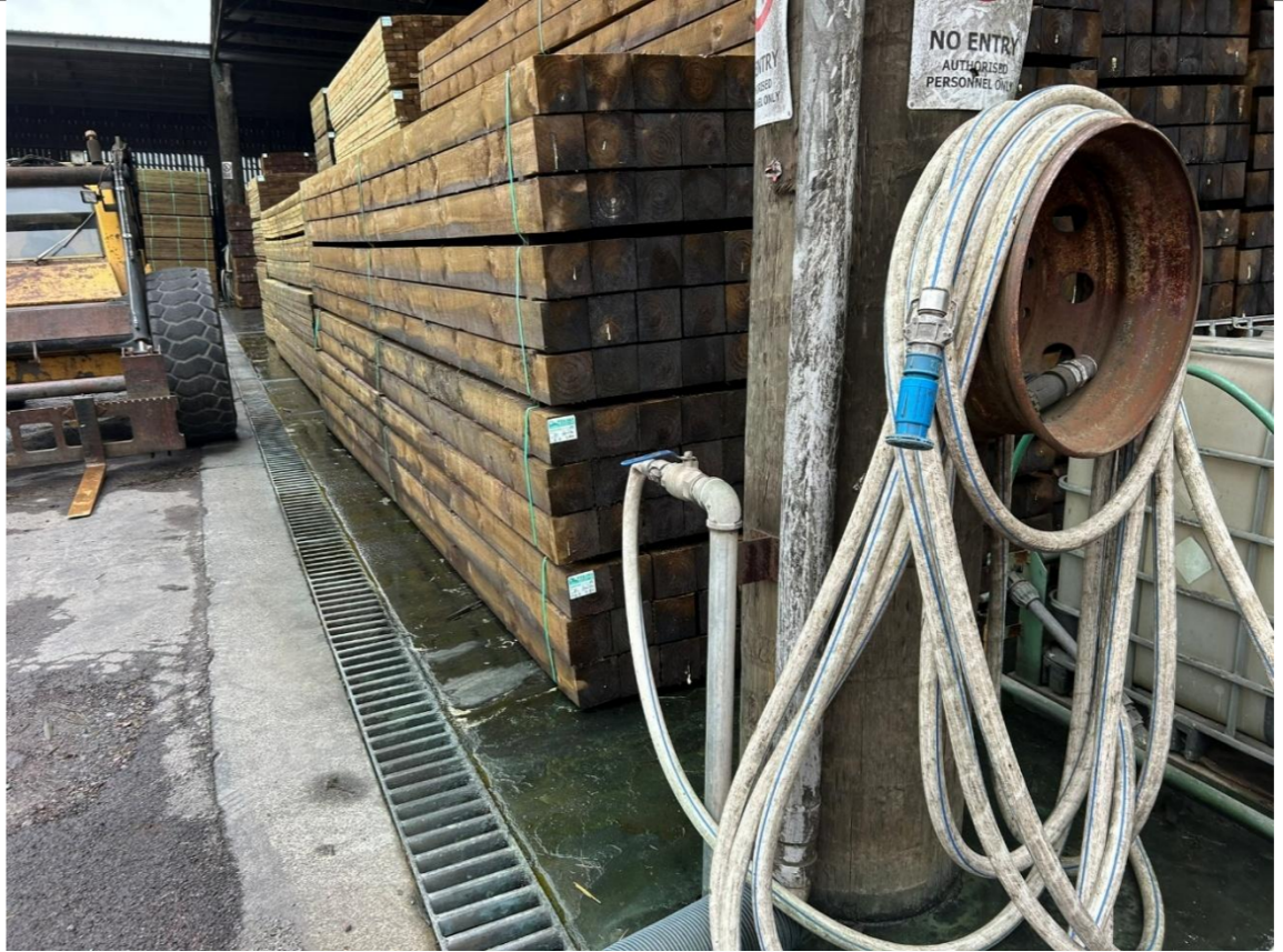
Photo 6: View of the bund capturing chemical runoff from the drip pad preventing staining beyond the drip pad.
