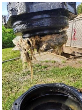
Further examples of blocked O/L pumps caused by Wet Wipes and rags.
