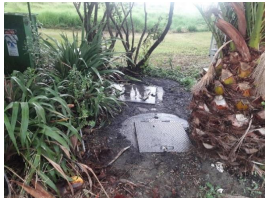
Donald Lane sewer manhole overflow (<math>< m^3 </math>)
