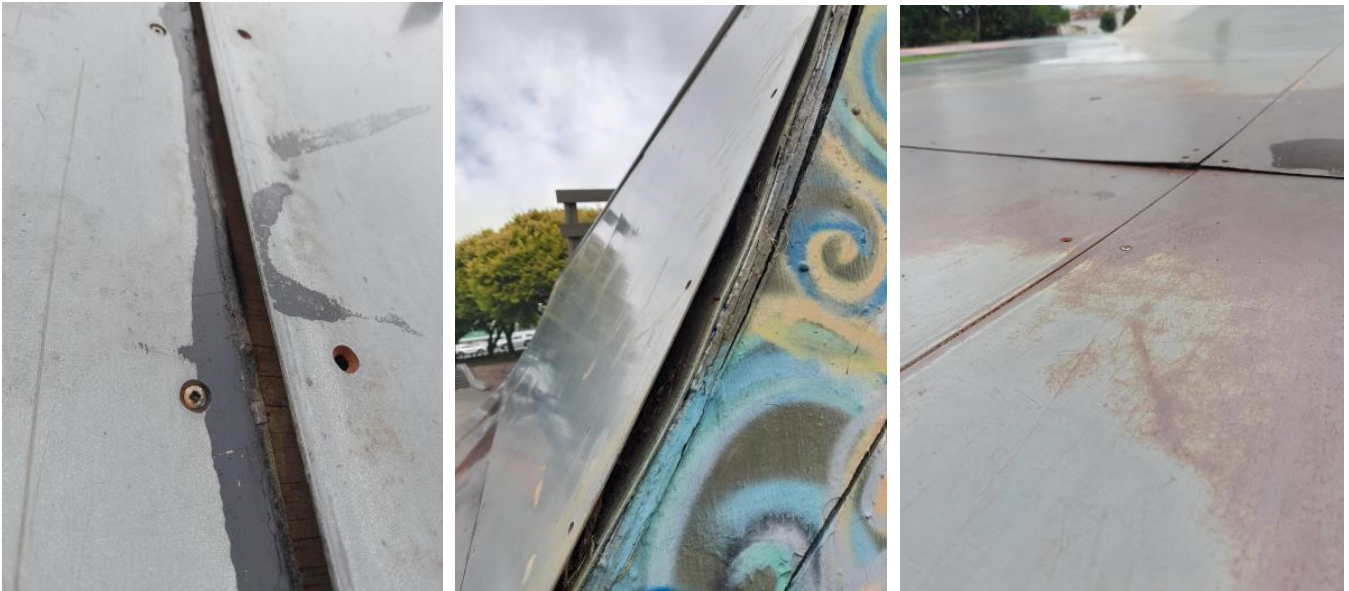
Steel plates have lifted on skate ramp
