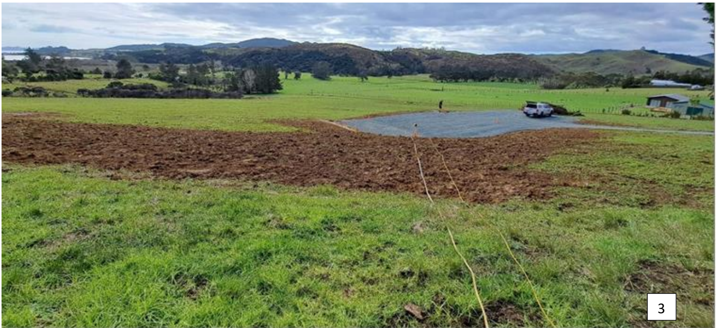
Photo 3 (above) showing the earthworks area as viewed from the Southern boundary corner.
