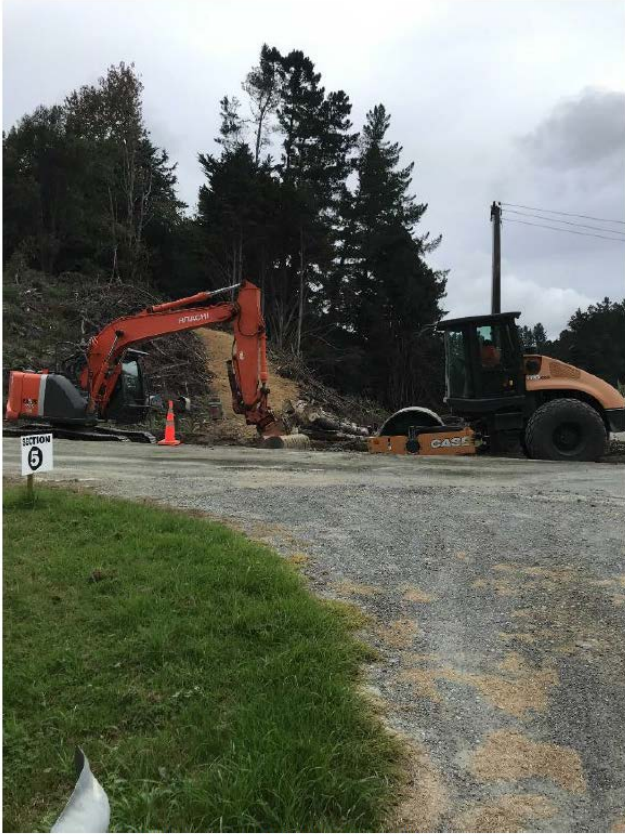
Figure 10: Section Five Bridge Undercut
