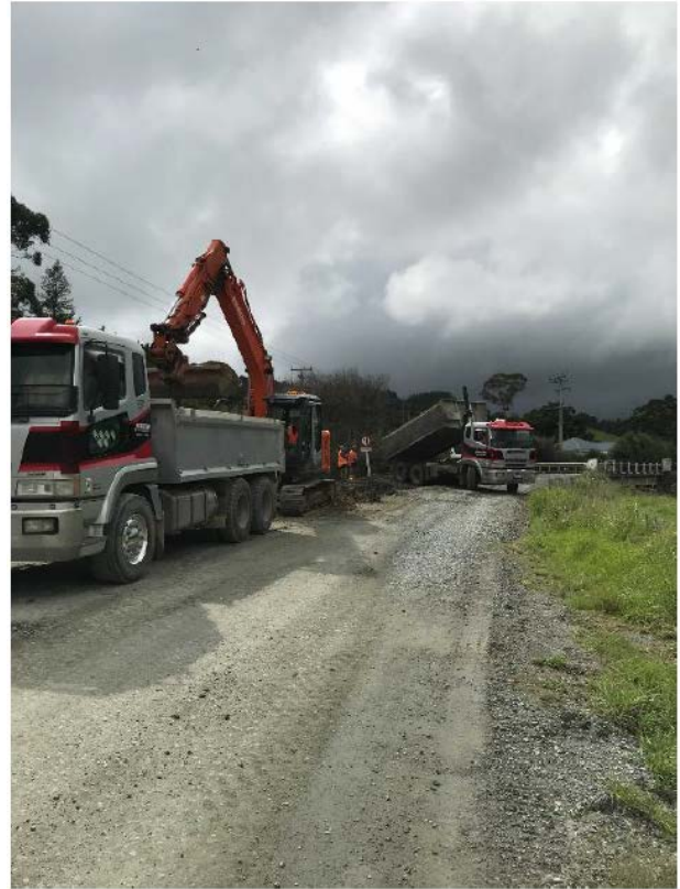
Figure 5: Section Five Bridge Undercut
