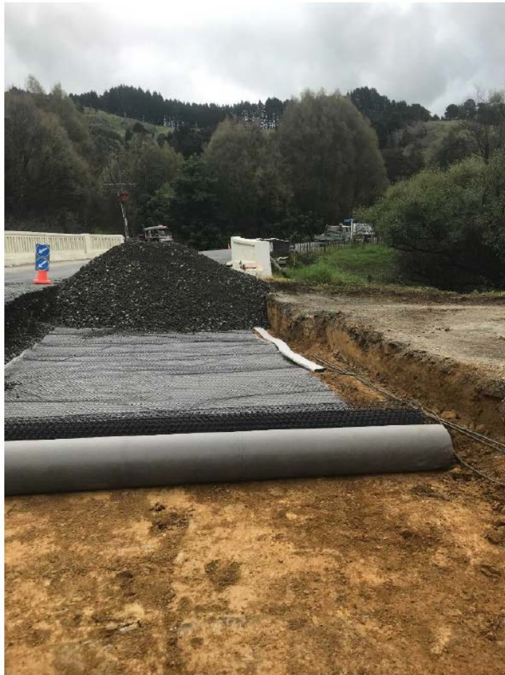
Figure 27: Section Five Bridge Undercut
