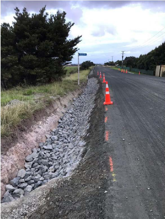
Figure 1: high risk shoulder with rip rap
