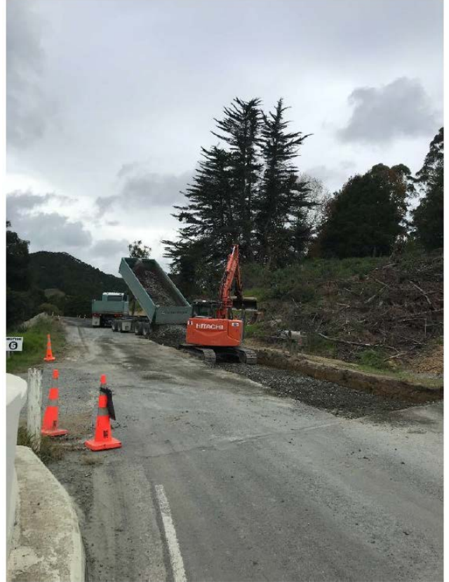
Figure 11: Section Five Bridge Undercut
