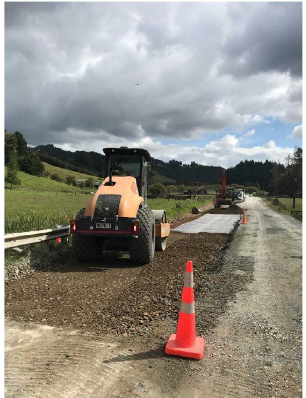
Figure 13: Section Five Bridge Undercut
