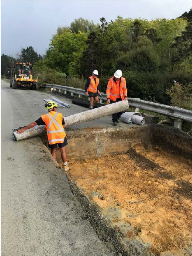
Figure 8: Section Five Bridge undercut
