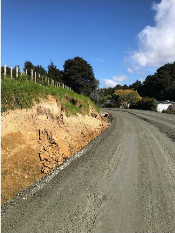
Figure 25: Section Four Storm Damage
