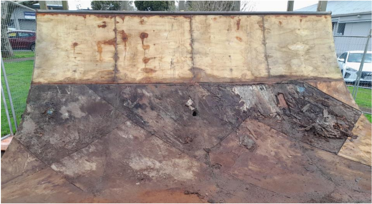
Kaikohe skate ramp metal plates removed exposing backing board
