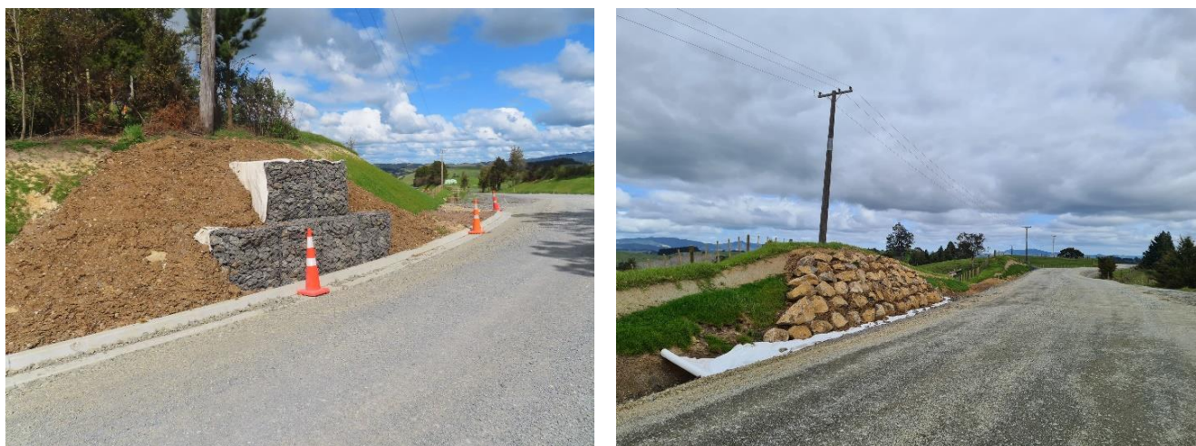
Figure 1) Additional retaining walls required.
