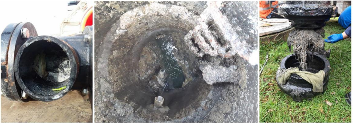
Wet Wipes – Mono Pump (L), Fat in Manhole – Kawakawa (center), Rag Ball PS Final - Kaeo
