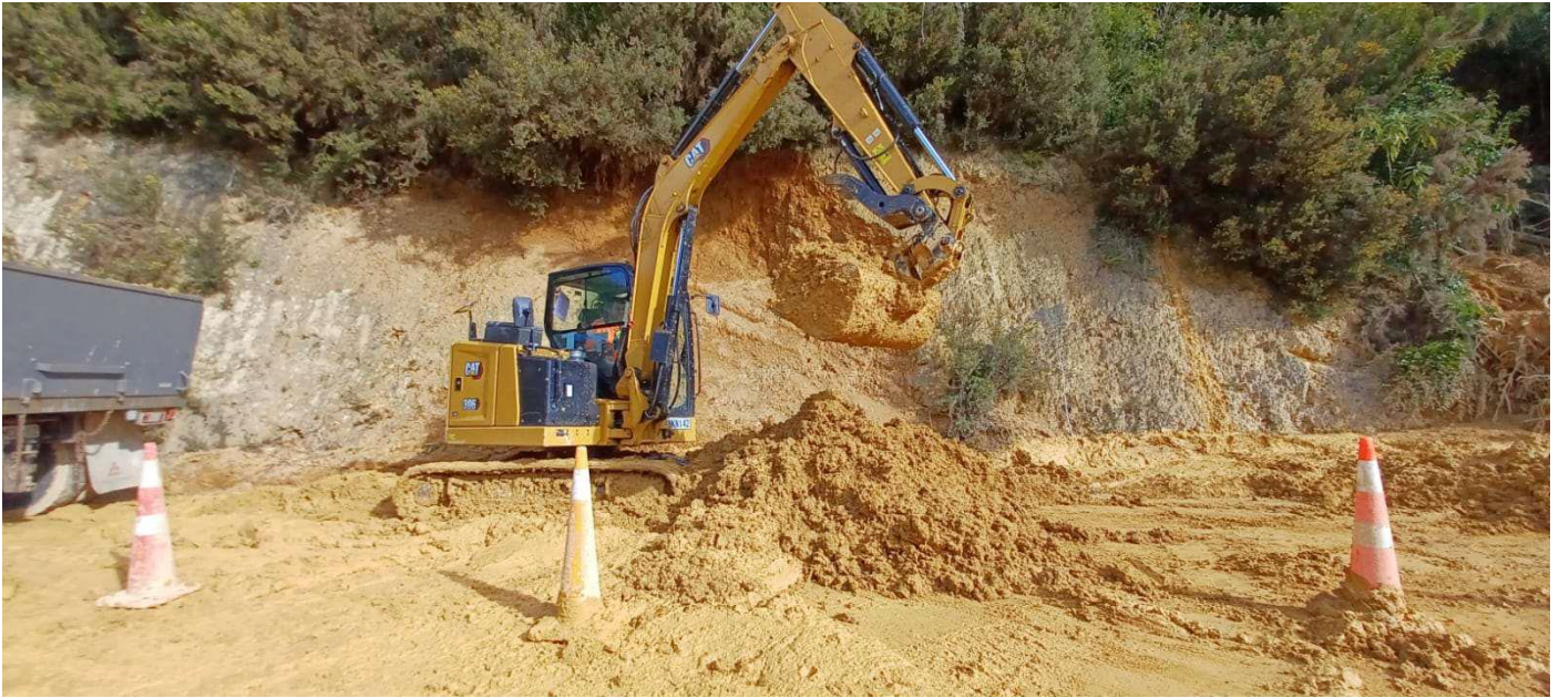
Step 4 – Load out stabilised clay into 6-Wheeler and cart to consent clean fill site.
