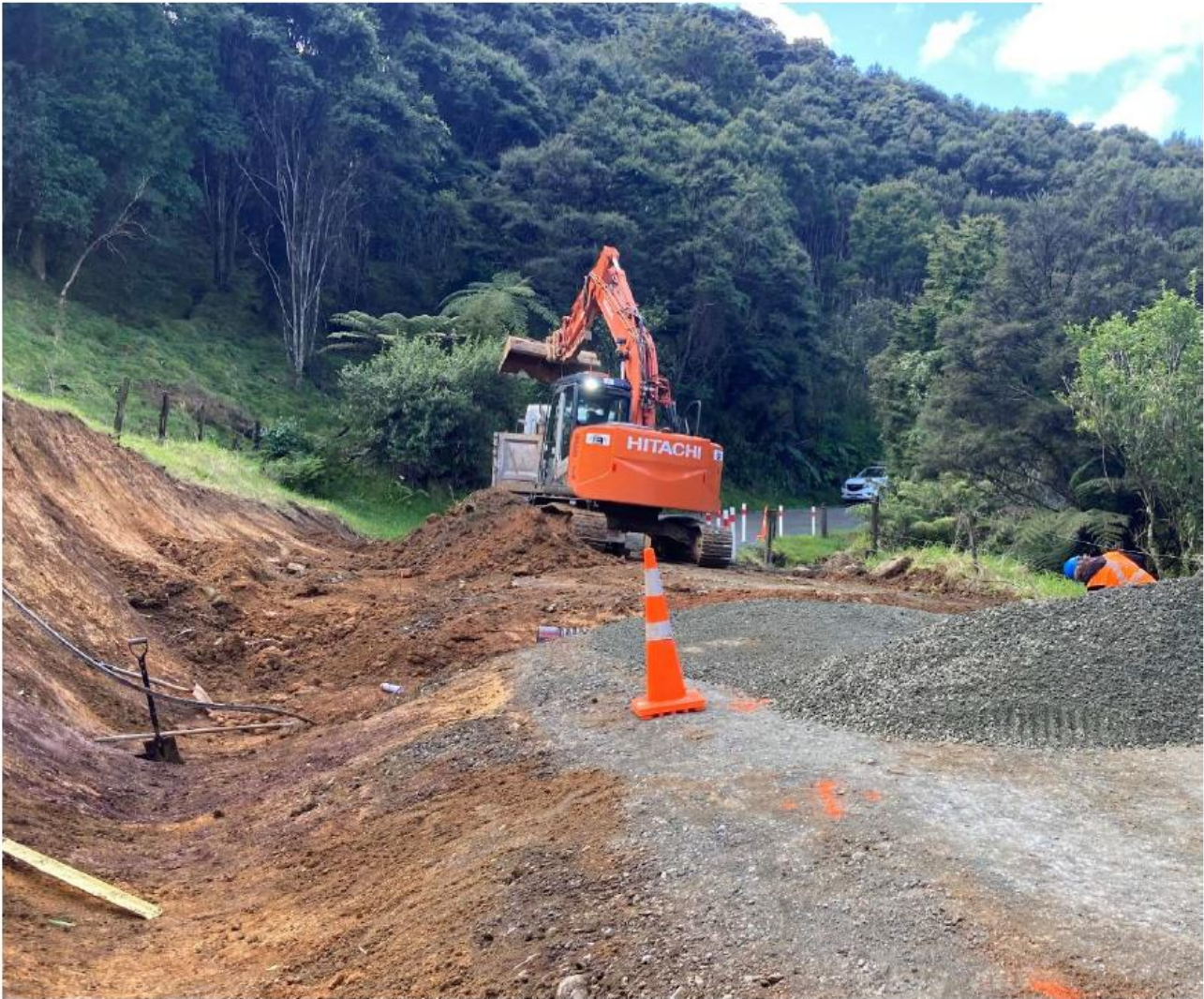
Culvert replacement on Kohumaru Rd where a pipe had come apart causing a Tomo.
