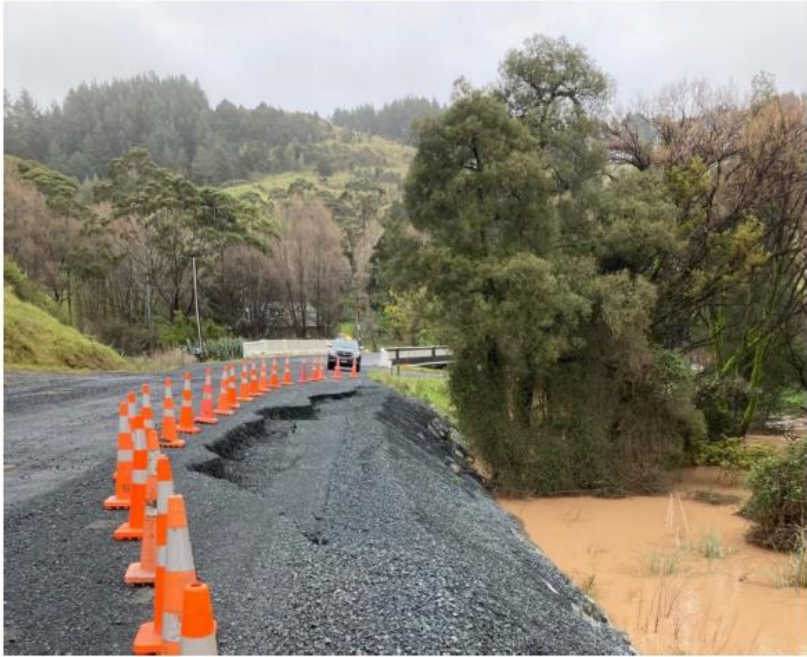
Underslip at Peria Road (near Wells Rd) programmed to be repaired this month.
