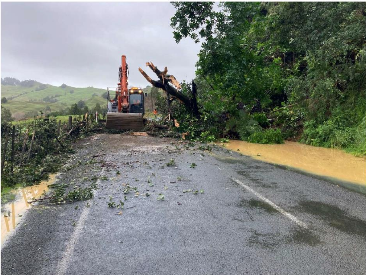
Emergency Callout to Broadwood Rd, part of the alternative route for the SH1 Mangamuka Gorge closure.
