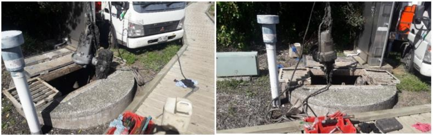
PS 3 Whatuwhiwhi showing ragged up pump following heavy rain event
