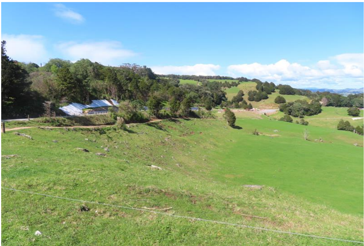
Figure 5) Site office view showing the top end of Ruapekapeka Road physical works in progress
