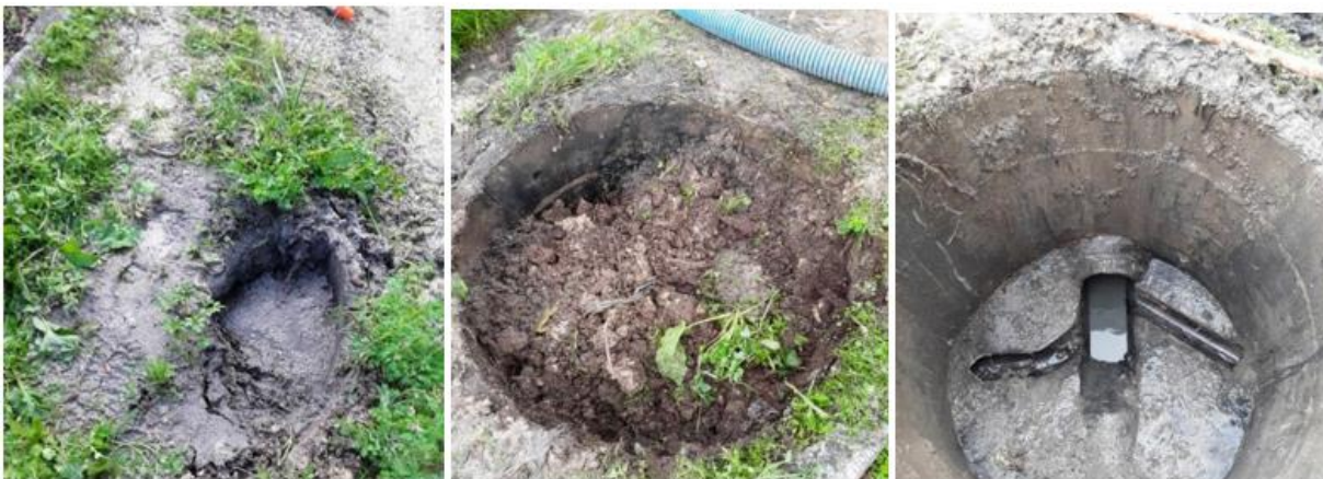
Buried and Filled Manhole – Rayner St, Kawakawa
