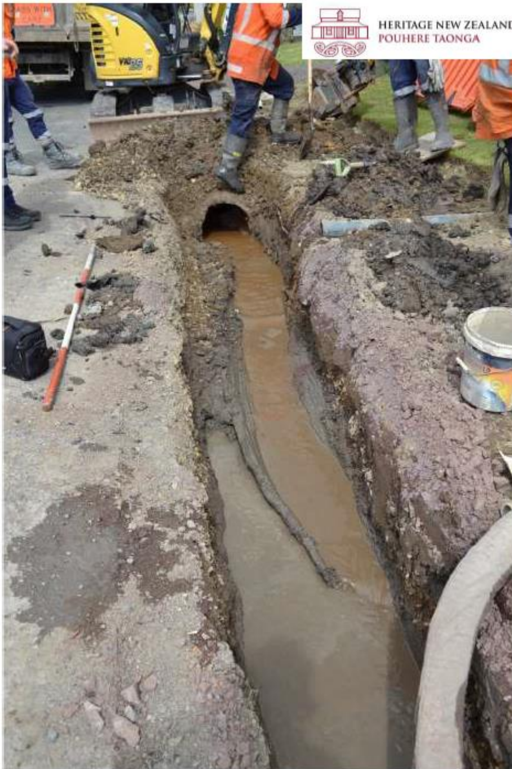
Figure 6: Once the Ventia team opened up the blocked concrete pipe culvert, the water flowed out and through the wooden item. This suggested that the item was part of a rotted tree laid in the swale drain that would have run alongside the old road and assisted in the transportation of water away from the adjacent properties. The lack of any construction adzing and the 'kink' in the item (visible here) confirms that that this was not built and would not function as a waka. It does however function as a culvert as is clearly visible here.
