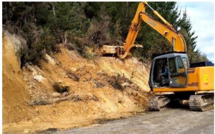
Ngapipito Rd – Slip clearing within site after 23 rd weather event.
