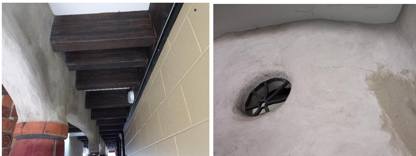
Hundertwasser Toilets with cracking in plaster work and wooden beams pulling away from neighbouring building
