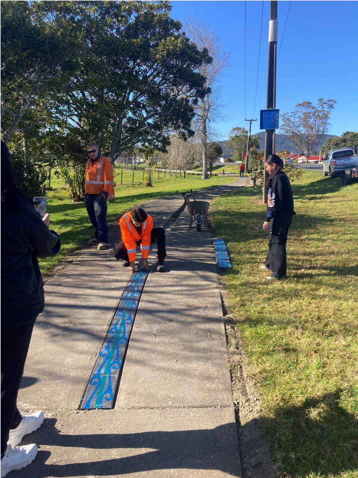
Franz Wagner, FNDC Project Manager, helping with the final tile installations on the Te Hiku Shared Path project.
