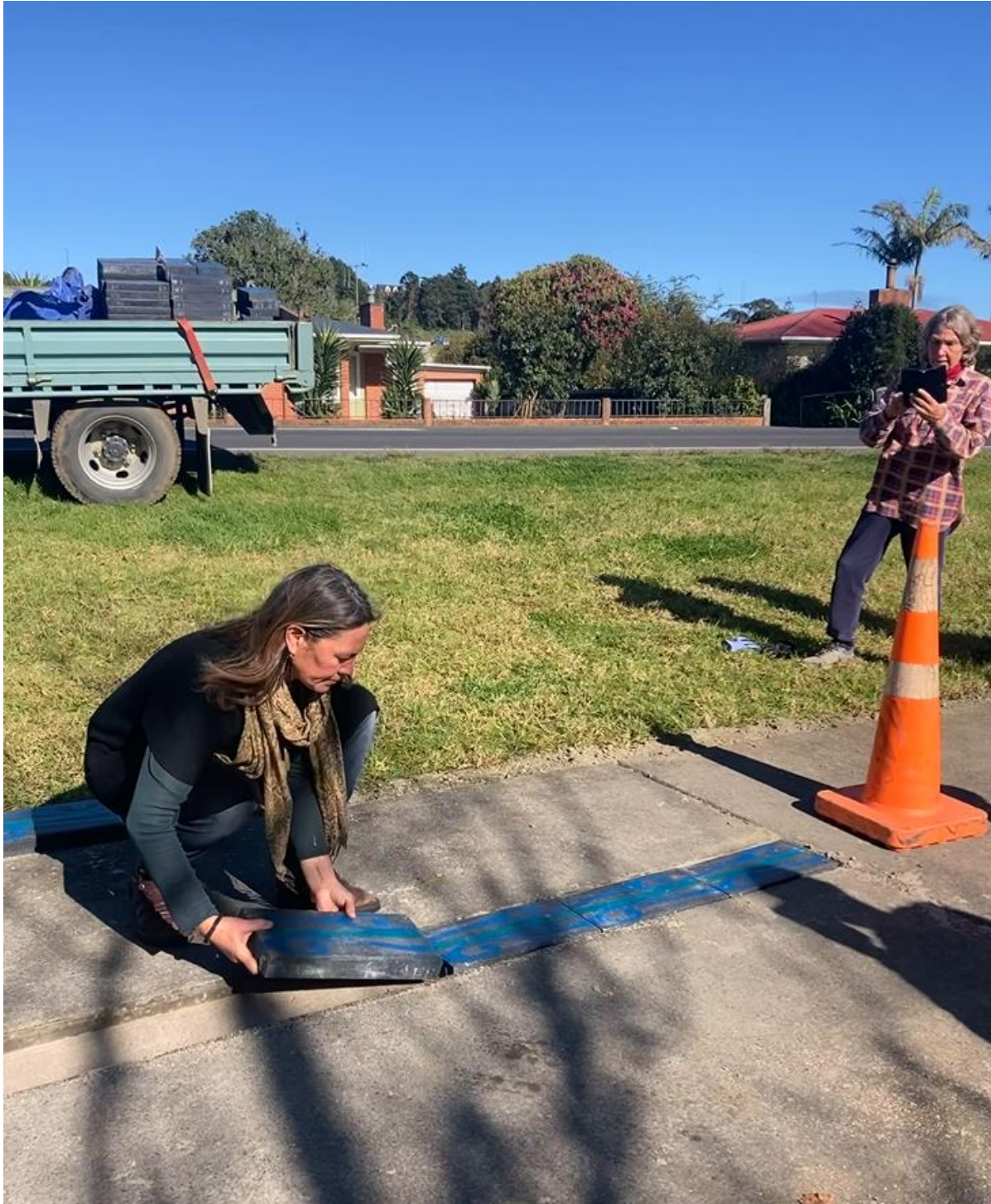
Waikarere Gregory, installing tiles hand painted by iwi representatives, the final stage of the Te Hiku Shared path, Kaitiaia.
