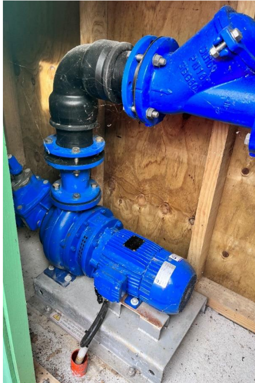
Figure 18 : Backwash water supply pump
