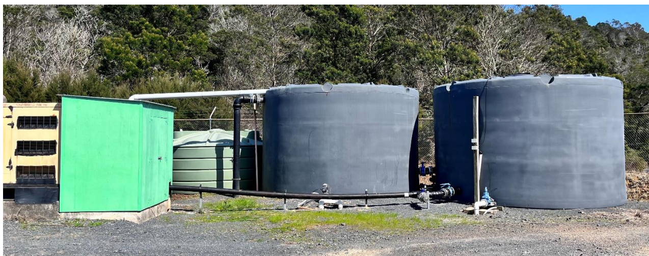
Figure 15 : SBR Receiving Tank 1 (Left) & Tank 2 (Right), with pressure filter charge pump house (far left)
