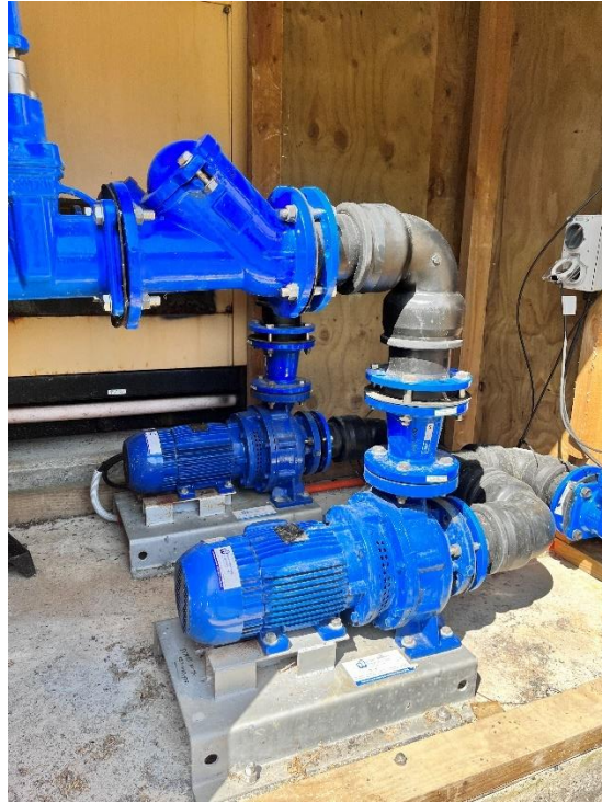
Figure 16 : Pressure filter charge pumps (P-001 A/B)
