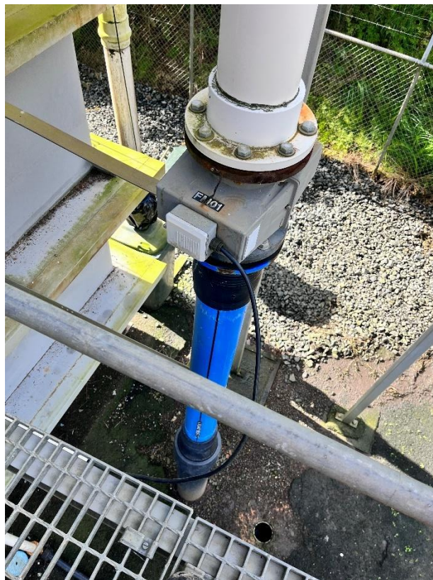
Figure 4 : Inlet rising main and incoming effluent flowmeter FM01.
