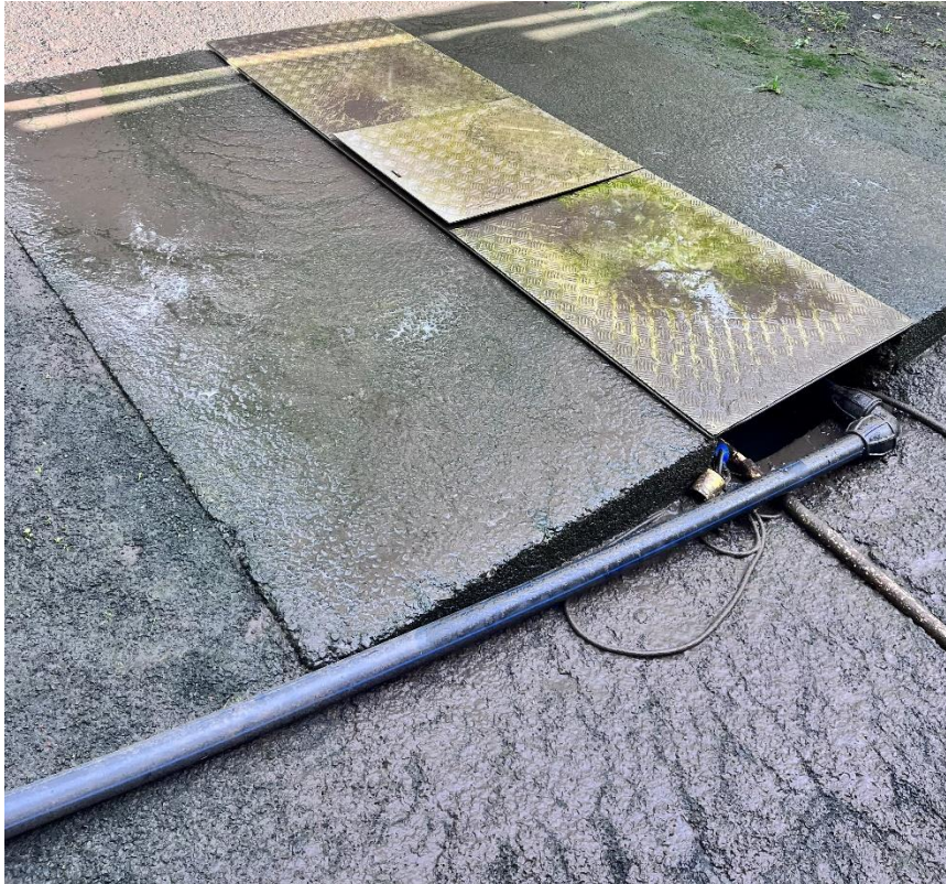
Figure 3 : Plant waste sump
