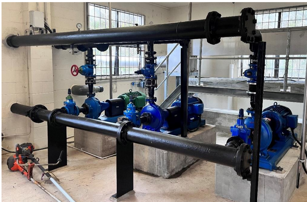
Figure 23 : Borehole Disposal Pumps
