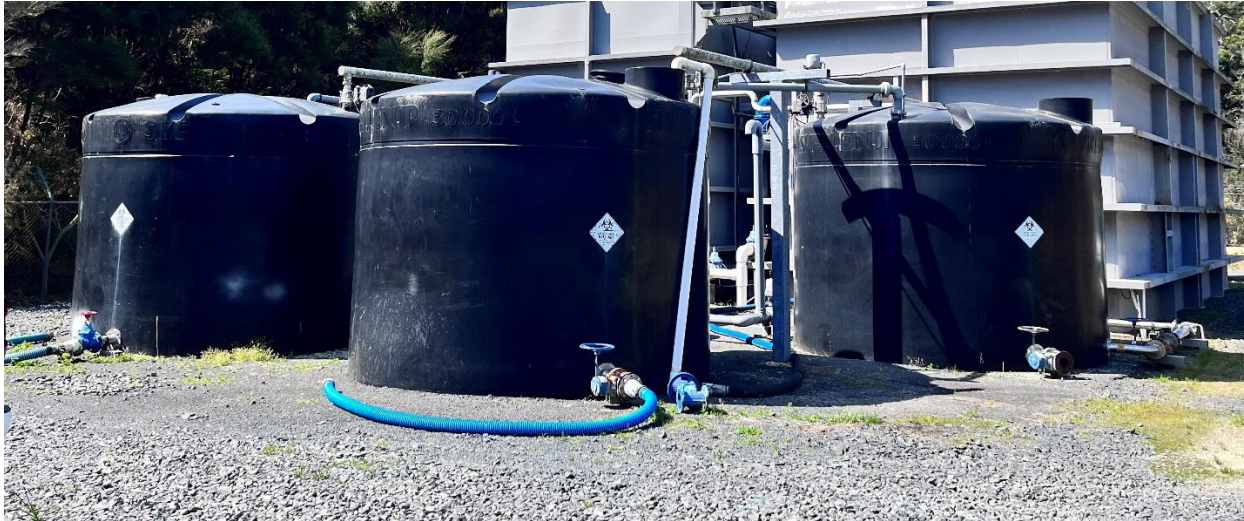
Figure 24 : Sludge handling system
