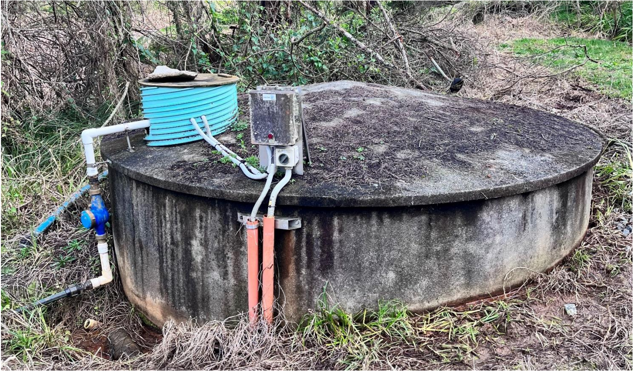
Figure 12 : Leachate Storage Tank (TK-009)
