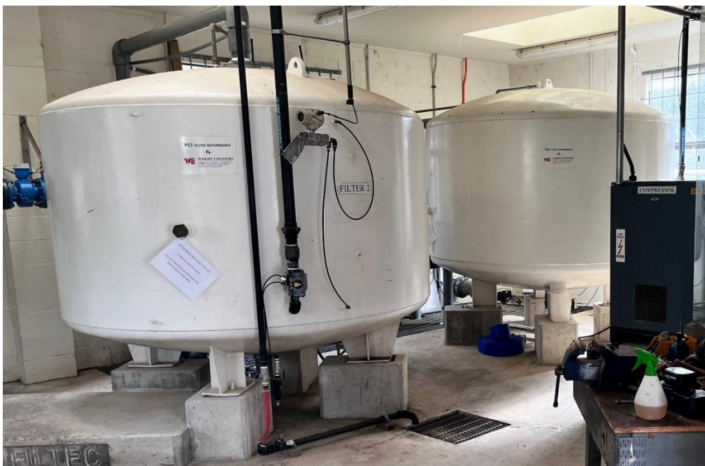
Figure 19 : Pressure filters 1 (foreground) and 2 (background)
