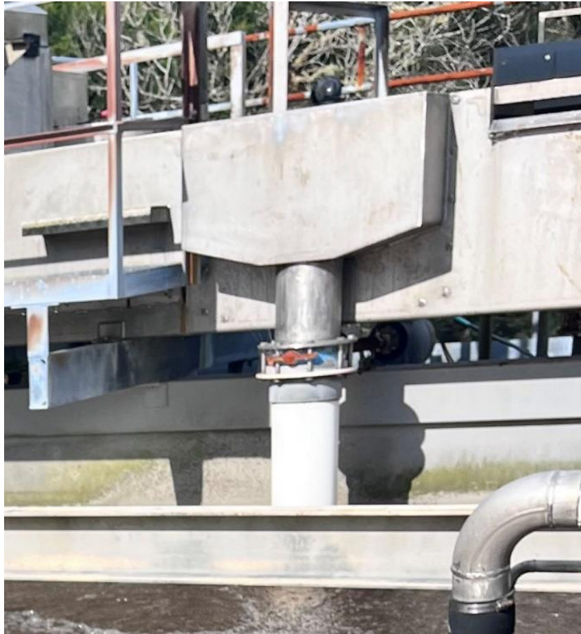
Figure 8 : Weir box influent splitter (T-05) and valve IV01 at inlet to SBR 1
