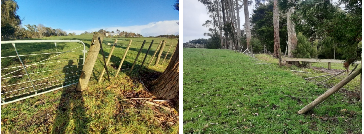
Lily Pond Lane Reserve - damaged fencing
