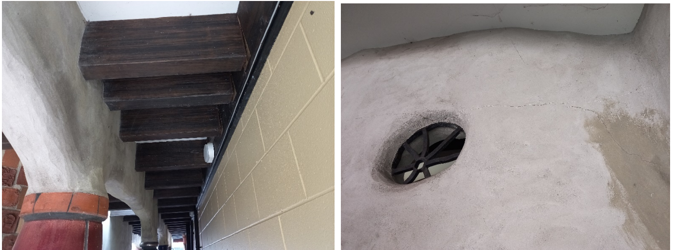
Hundertwasser toilets - cracking in plaster work and wooden beams pulling away from neighbouring building
