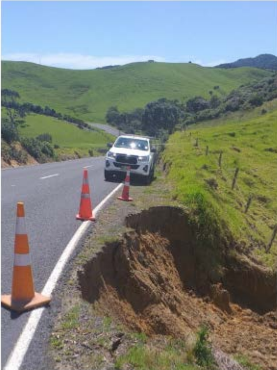
Rawhiti Rd South – Under slip
