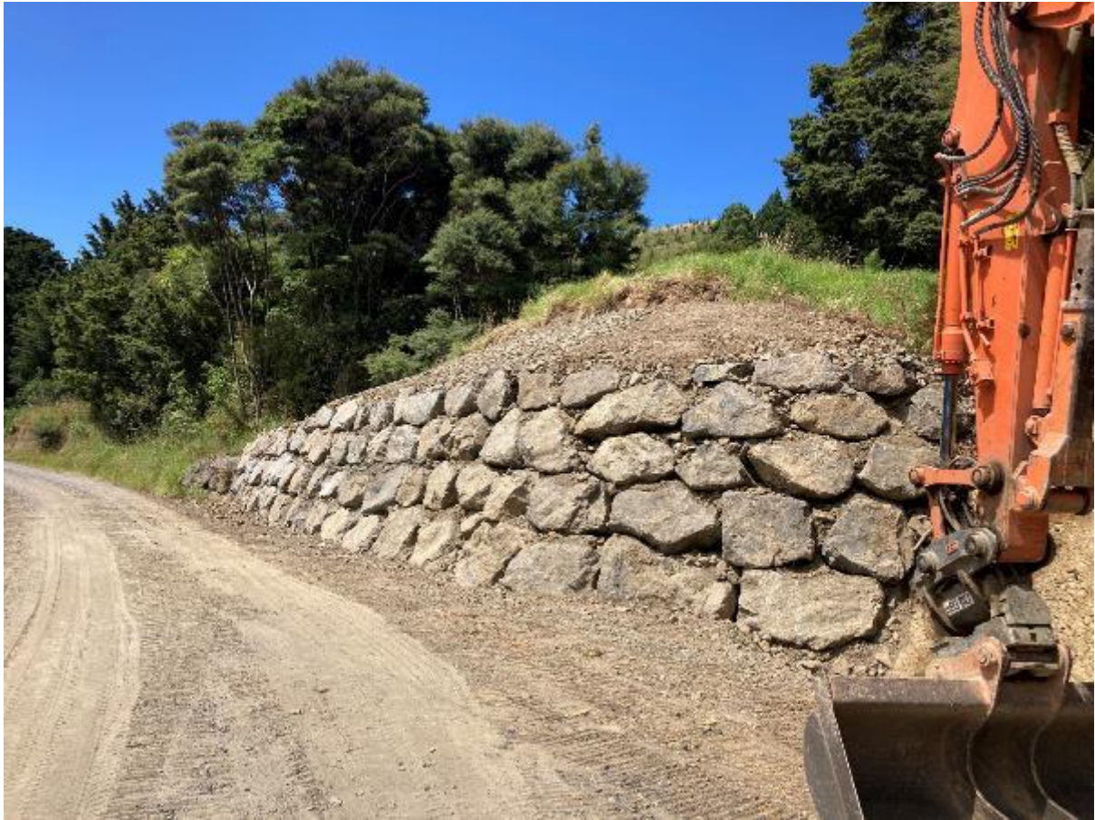
Diggers Valley Road Storm Damage Repair
