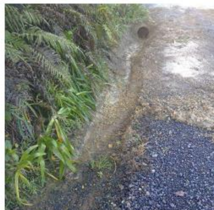
Hupara Rd – Routine culvert end clear with small section of water tabling to ensure adequate drainage.
