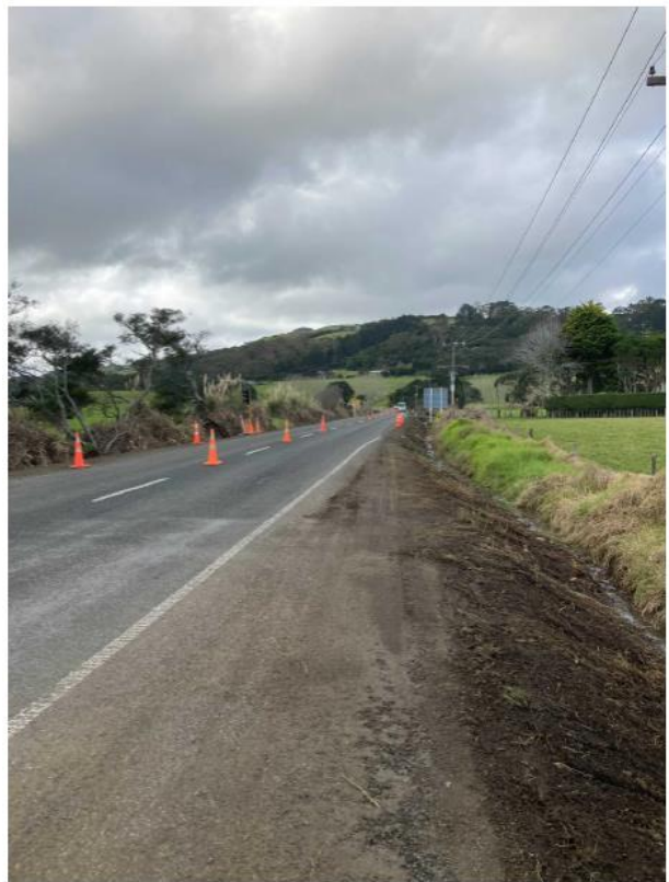
Figure 9: Kaitaia Awaroa Rd Pre Reseal Watertabling
