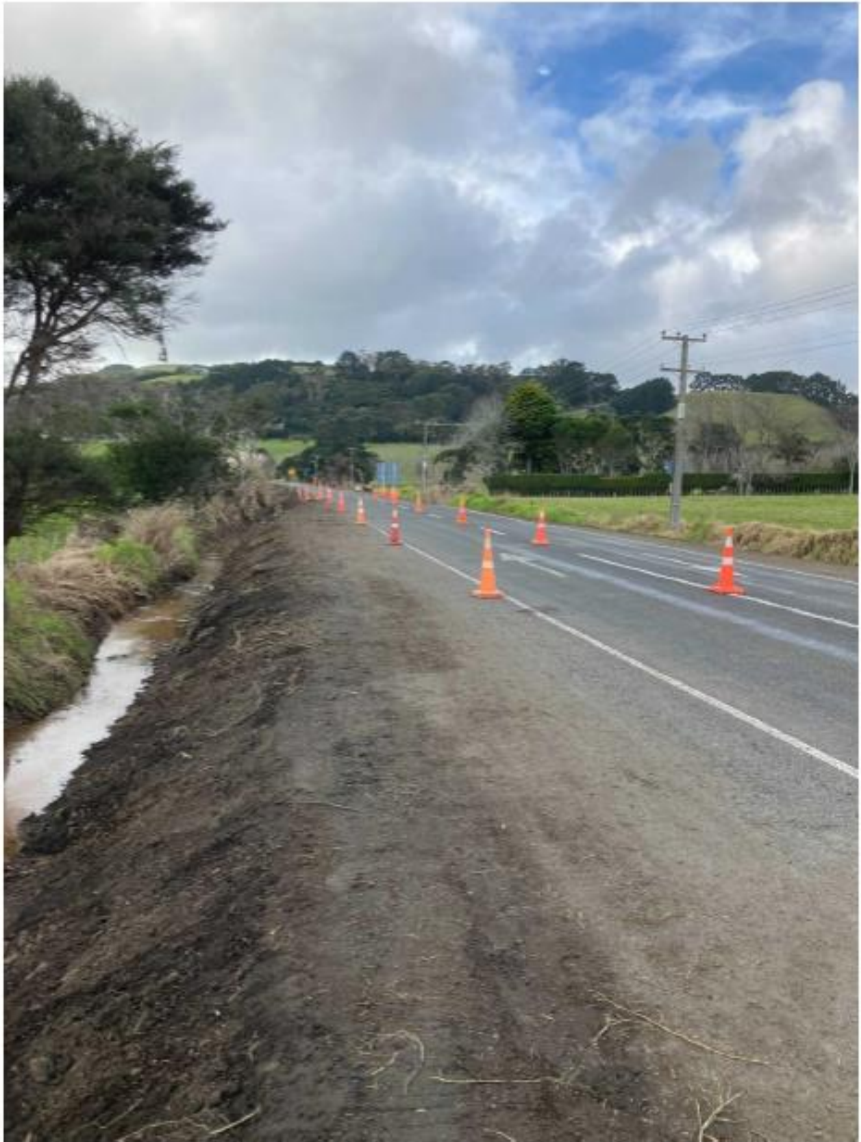
Figure 10: Kaitaia Awaroa Rd Pre Reseal Watertabling
