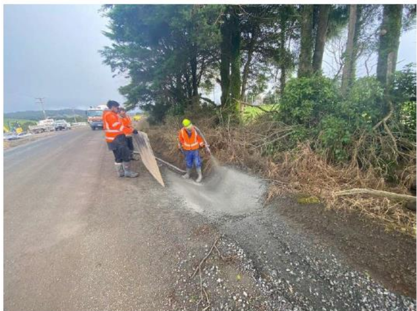
Pungaere Rd – Concrete pumping a new swale in a high discharge area
