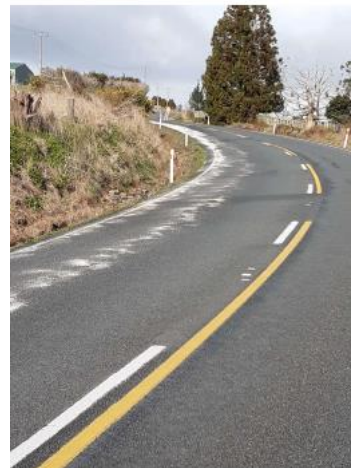
Diesel Spill rung in through the RFS System – Old Bay Rd
