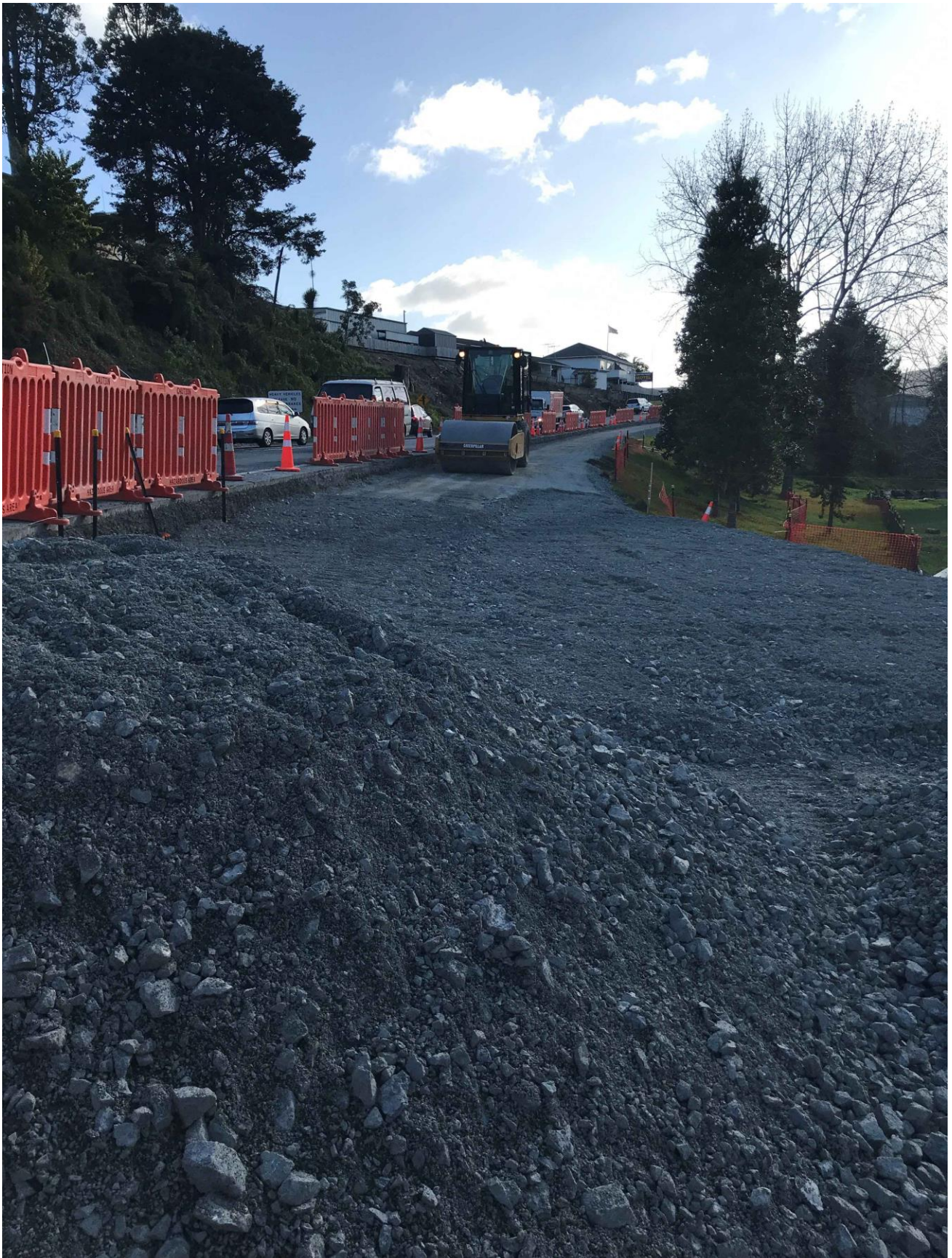
200903_2: The shoulder being widened to construct the temporary intersection to allow the new intersection to be built. In a few weeks, this will be a traffic lane(s).
