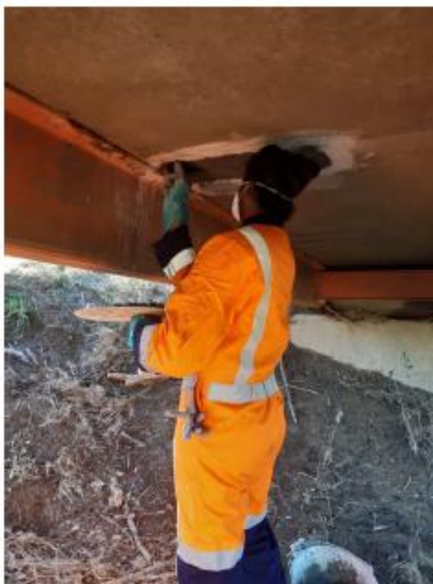
Jash our Renewals Manager trialling the application of Sika Products on the General Bridge Repairs Contract
