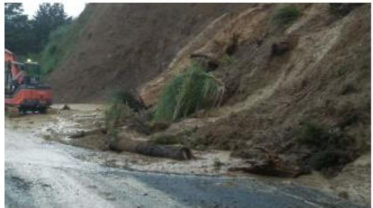
Pipiwai Rd – Slip continuing to fall in rain events post July storm
