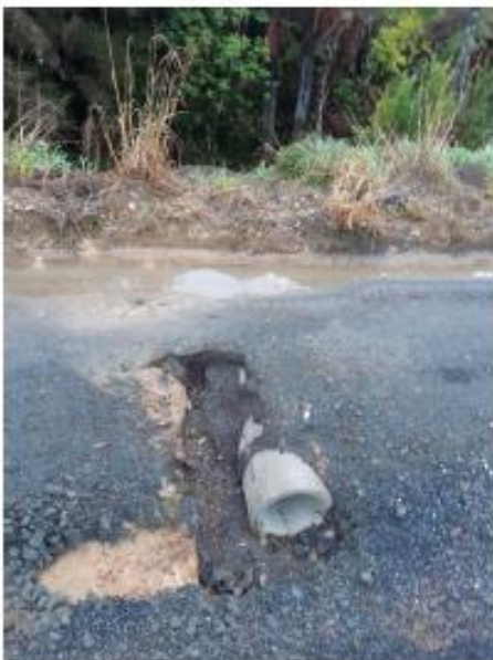
Culvert Wash out
