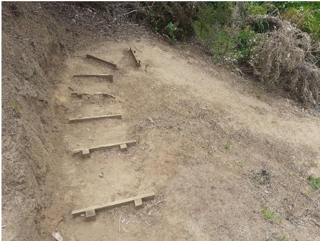
Current condition of steps on Te Araroa Trail on FNDC owned reserve
