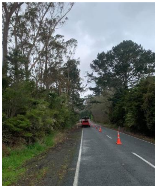
Site 10. RP 15865 – 15870: Removal of overextended Gum tree branches which were encroaching onto the highway
