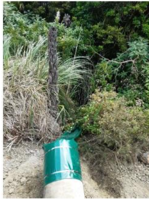
Cabbage Tree Bay Rd – Culvert sock installed on end of pipe extension following storm event
