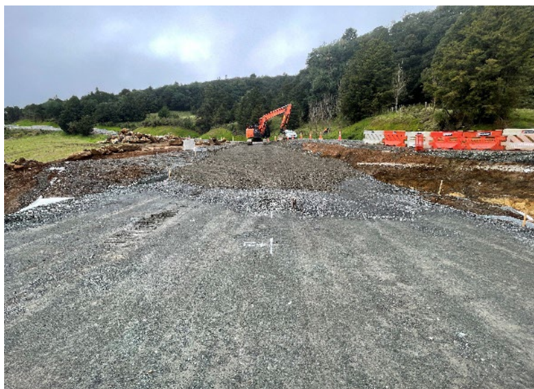
Figure 1) Lifting the road over the 2.1 culvert with fill to tie in with existing road level.
