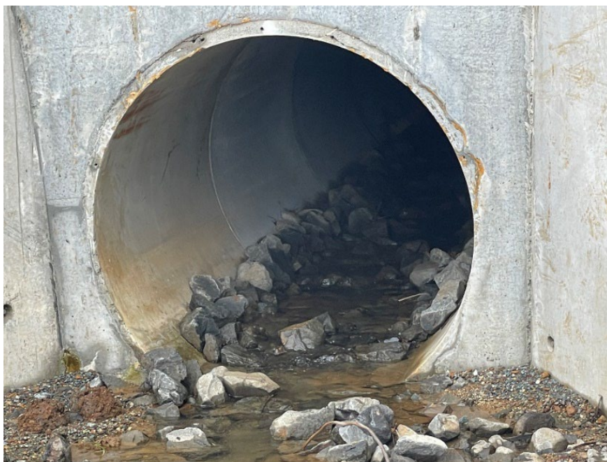
Figure 5) As part of NRCs consent conditions (NES-FW) the 2.1dia culvert required a fish passage. When working within waterways, fish passages are a requirement to allow fish to move unobstructed through the waterways.
