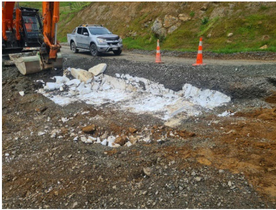
Figure 3) Polystyrene uncovered under the road where the new 2.1dia culvert was installed. This was an old method used for a lightweight bulky fill under roads. The extent of what was uncovered and what needed to be removed was more than the contractor anticipated. As you can see in the photo it was first discovered after scraping back the surface layers, and as they dug deeper to clear it out the extreme volume of material became evident.
