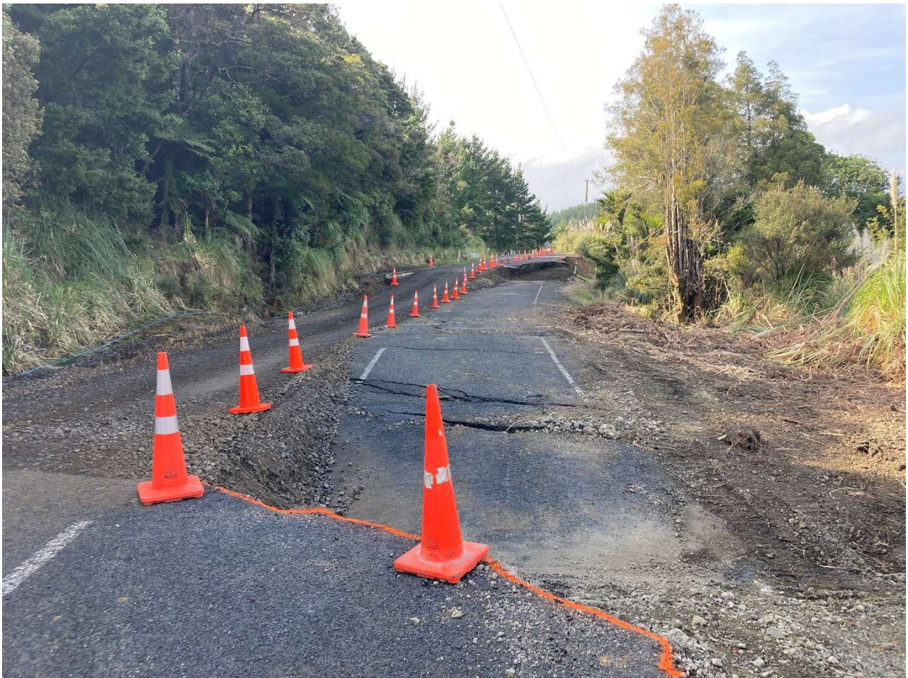
West Coast Rd (Motuti) slip opened to light traffic this month
