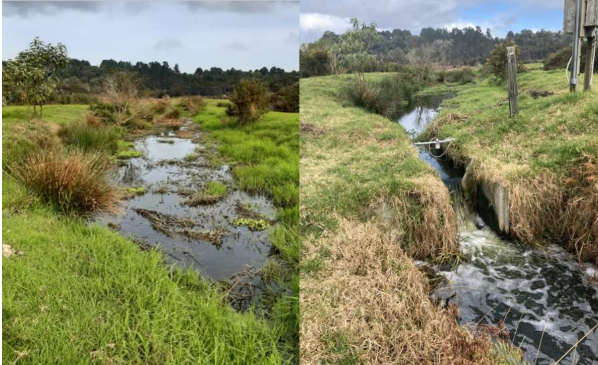
Figure 3-2 Constructed wetland system (left) and weir structure (right) located at the point of discharge at the Kaikohe WWTP. Image taken by report author 28/7/2021.
