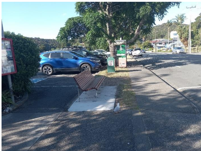
Williams Rd seat installation to eliminate potential trip hazard
