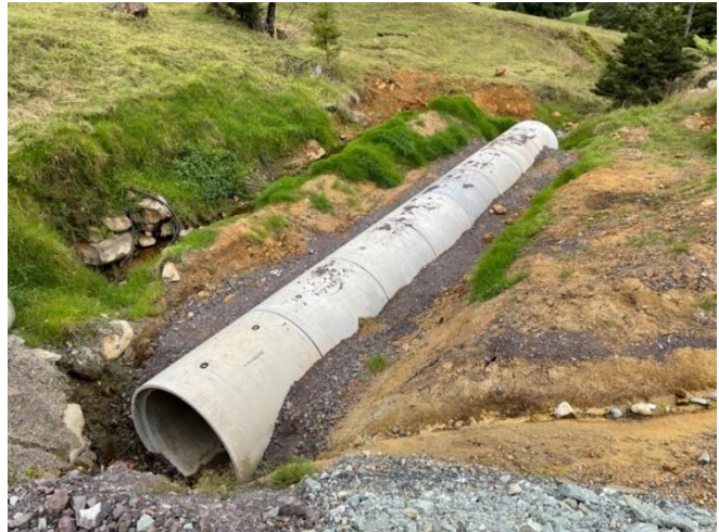
Culvert 2100 Ø in place awaiting the replacement to one section of pipe
