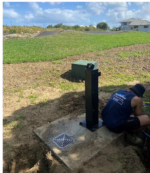
Water fountain at Pump Track
