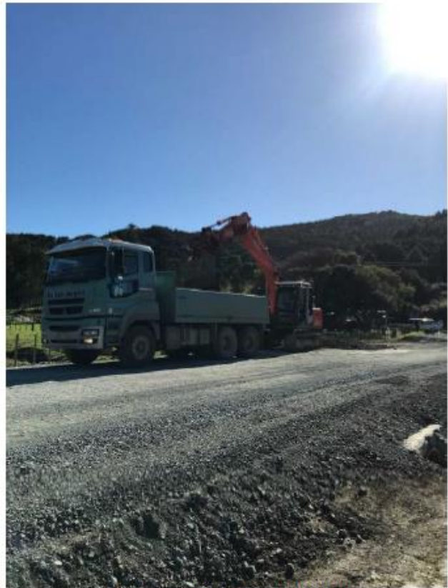
Figure 5: Section 5 Pavement Undercut
