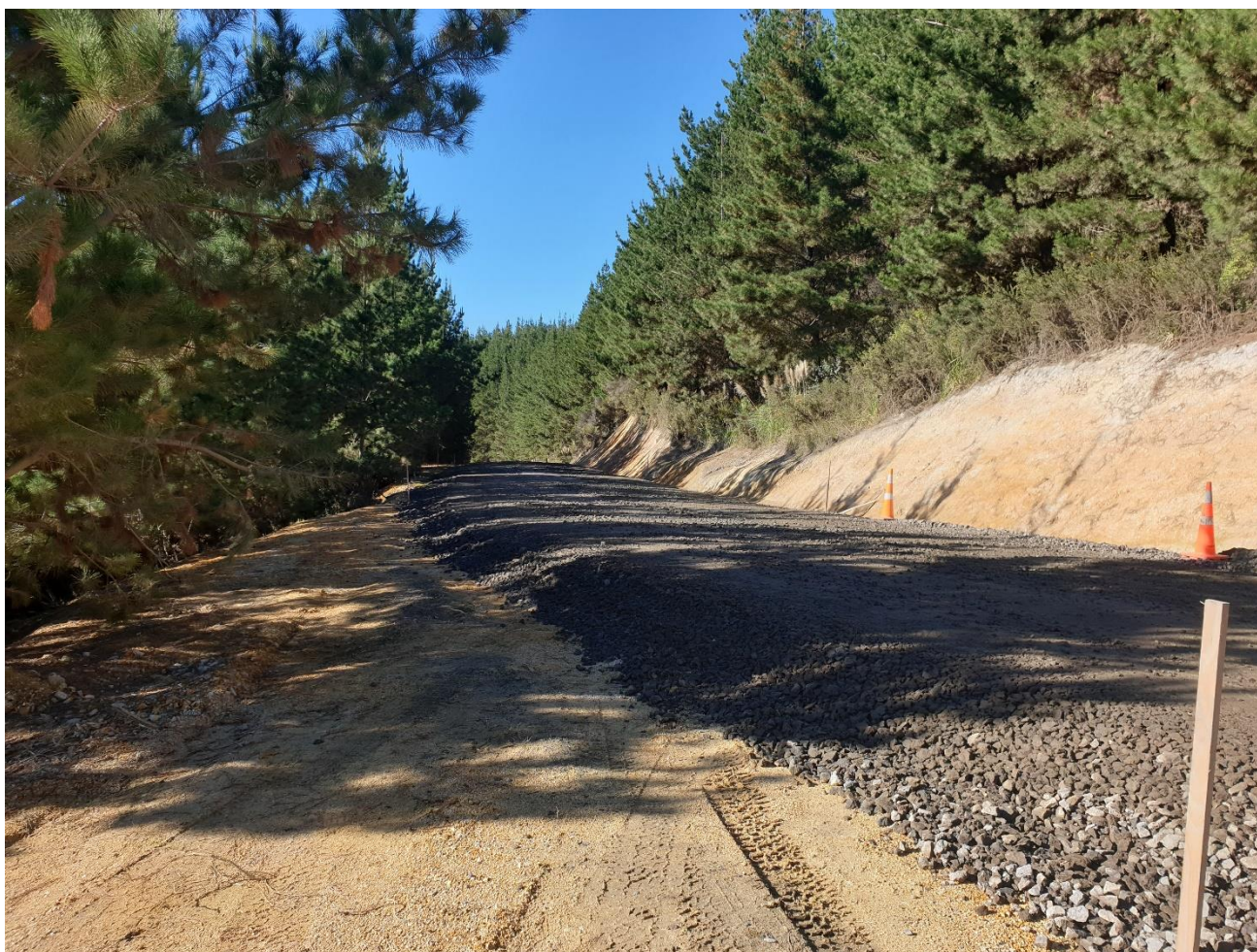
Subbase pavement layer has been overlayed and compacted on Sections 1, 2 and 3 at Ngapipito.
