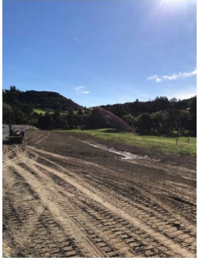
Figure 7: Section 5 Tip site fencing
