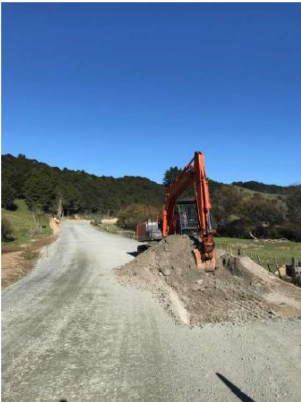
Figure 4: Section 5 Pavement Undercut
