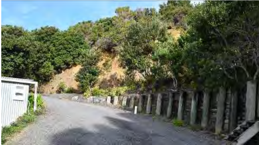
Photograph 6: A shot of the lower tier of several portions of retaining wall that are supporting the bank near the existing house. These are now largely subdued by vegetation when compared to their more explicit state in the photographs of Attachments Three and Four. A water tank sits near the entry to the main body of the property, just outside of view to the left of Photograph 1 and marked on Attachment One.
