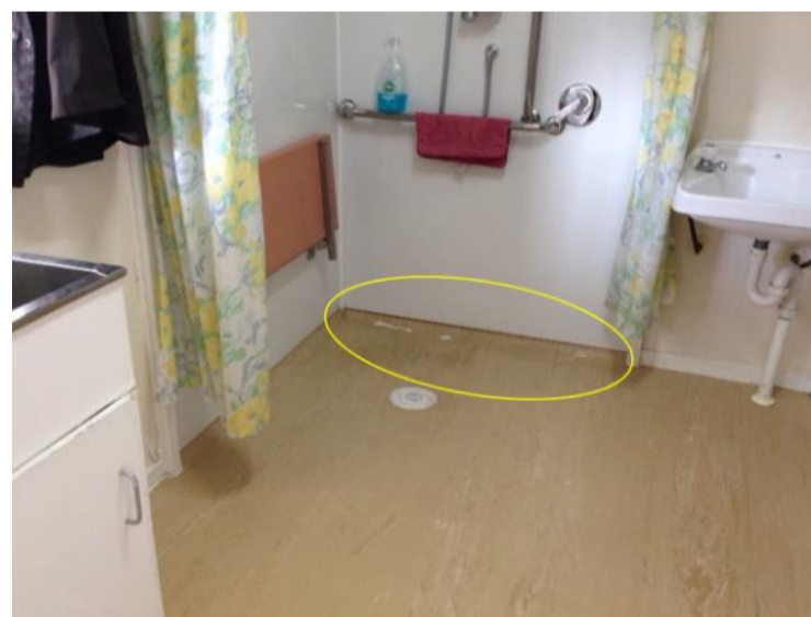
Unit 1, Horeke vinyl cracked along cove of wall
