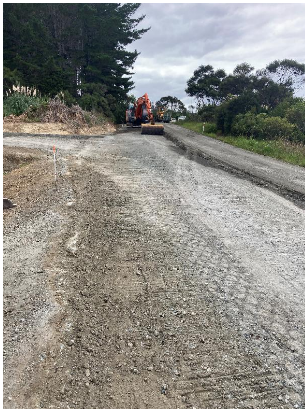
Figure 17: Kohukohu Rd Pavement Undercut
