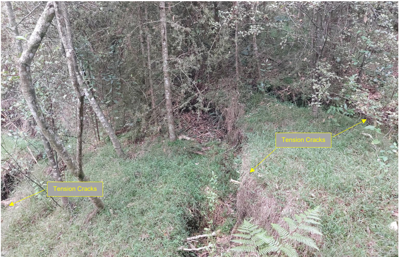
Figure 10: Photograph of the tension cracks identified on the northern slopes down to the Puketotara Stream.
