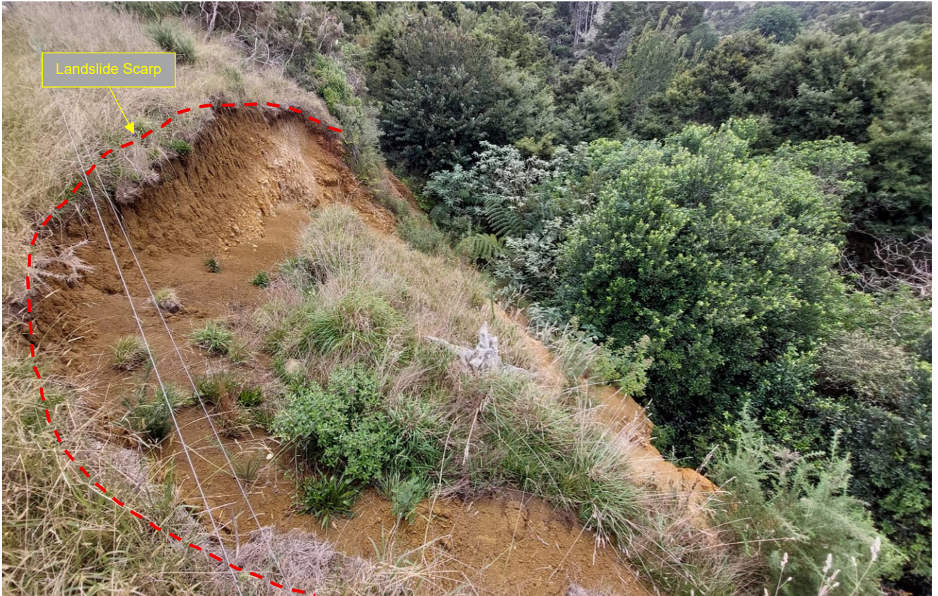
Figure 9: Photograph of the type of failure located on the northern slopes above the Puketotara Stream.
