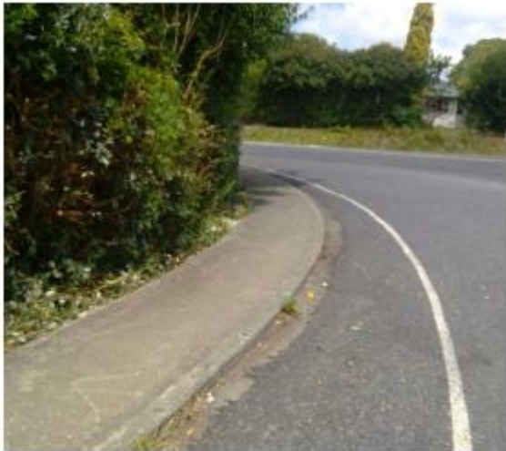
Riverview Rd/Landing Rd Intersection – Footpath Vegetation trimming
