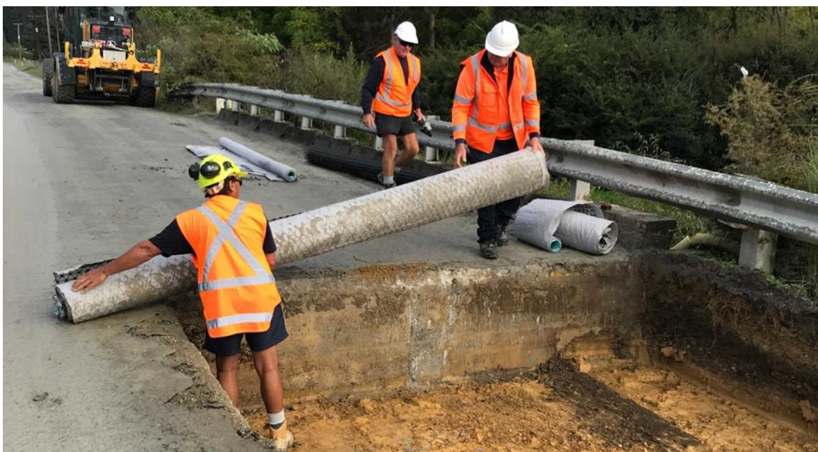
Bridge undercut at Peria on Section 5
