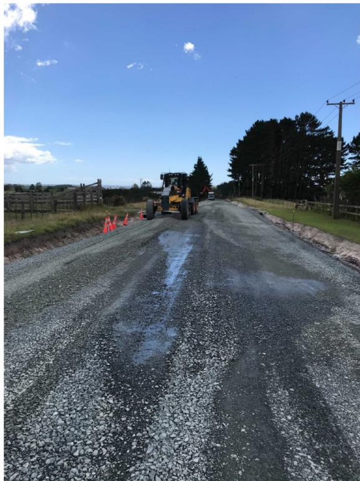
Figure 3: Water flow up through basecourse requiring subsoil drainage
