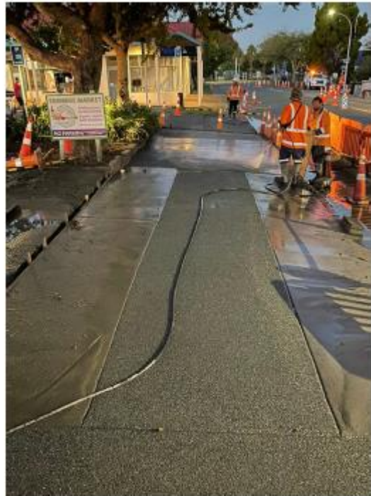
Hobson Ave – Footpath Exposing – Not delineation treatment designed to make it clear for pedestrians where to walk at vehicle crossings.
