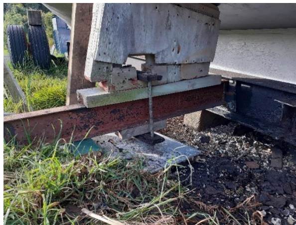
Extent of repairs required to the boat trailer prior to re-launching – Te Hue Bay
