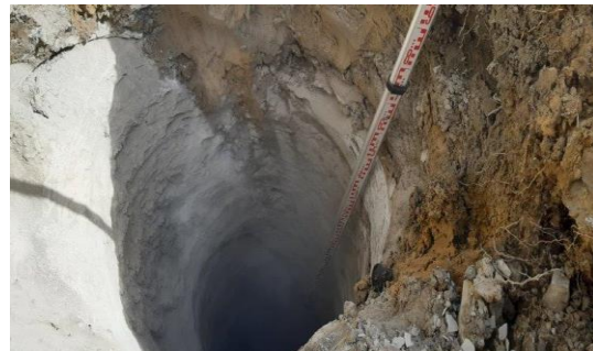
FNDC Contract 7/22/159 - EW Slip - Fairburn Rd Pole installation progressing through hard rock
