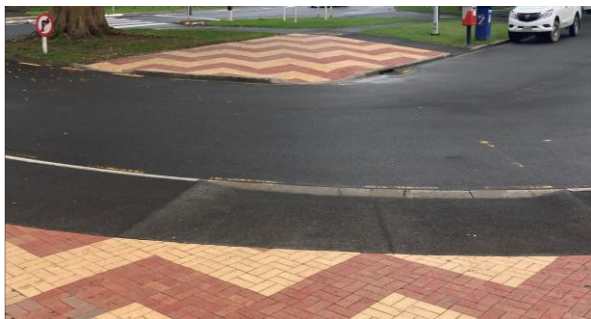
FNDC Contract 5/19/101 - Te Hiku Te Ahu Loop Running Track & Boardwalk - NuBrick extension to the Te Ahu Entrance
