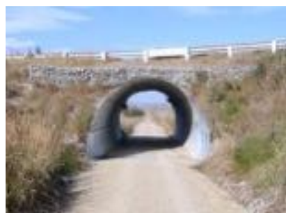
Underpass on Otago Central Rail Trail, Otago Region (courtesy of OCRT Trust)
